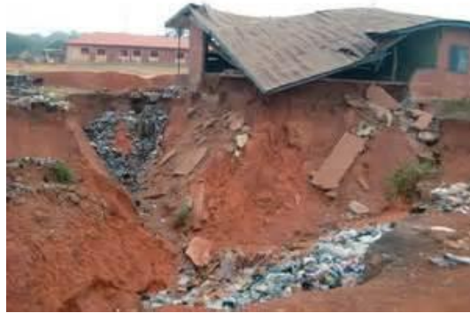
Plate 2. Eroding building along the gully advancement path influence by slope
